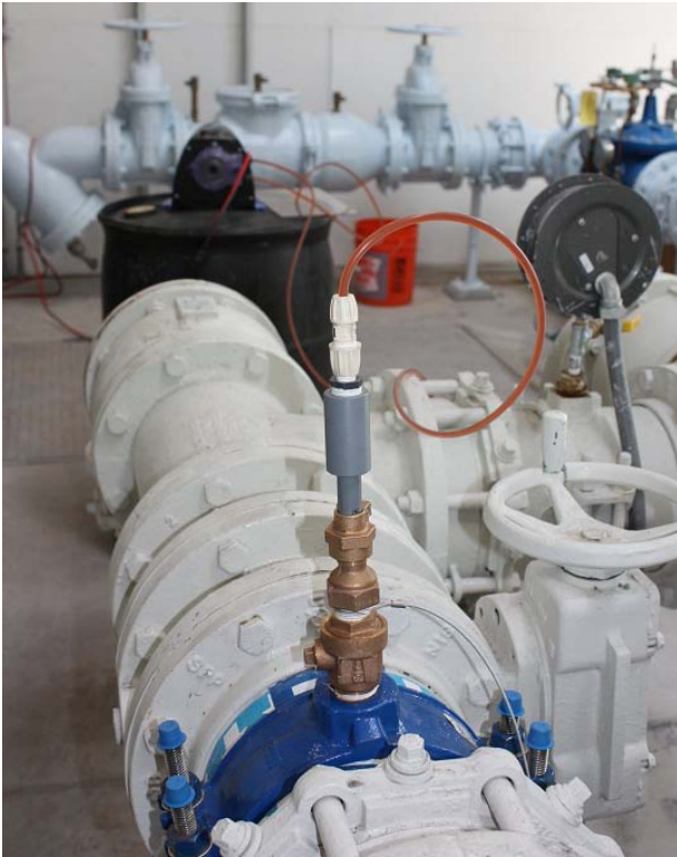
Figure 1: Ferric Chloride Injection Port and Pump at Well 4
